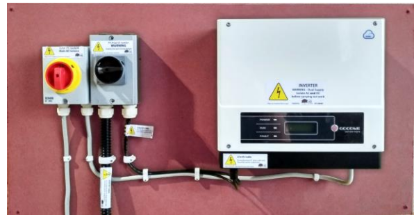
Figure 15: Installed inverter with electrical isolators
